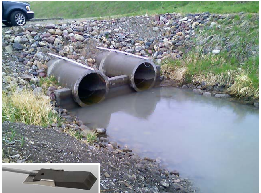
AVFM Ultrasonic Sensors Mounted at the Bottom of 36" Concrete Culverts
