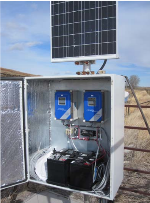
Solar-Powered AVFM Area-Velocity Flow Meter Electronics Installed in Panel with Batteries
