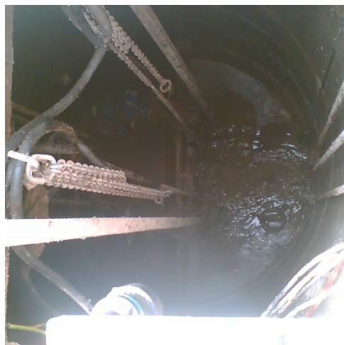
A typical wet well installation.
