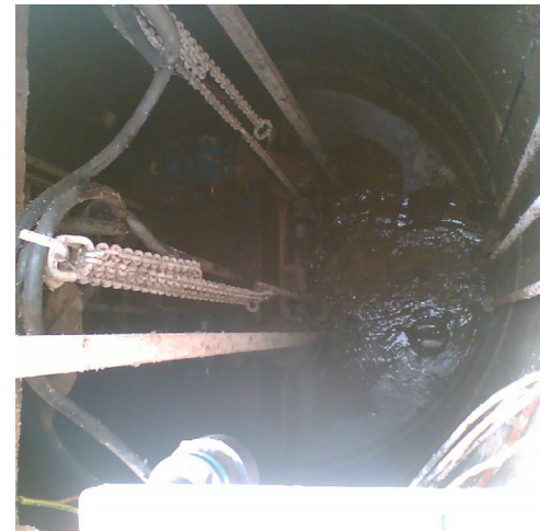
A typical wet well installation.
