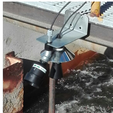
MicroFlow and dBMACH3 in a wastewater application
