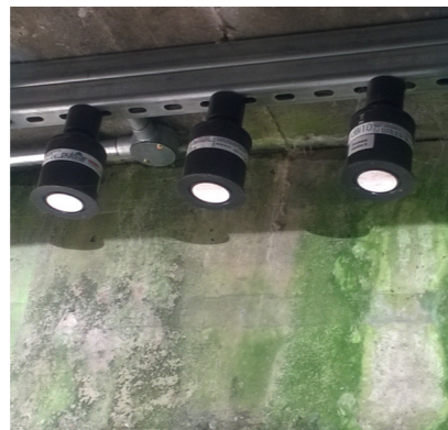
3 dBi HART transducers Monitoring Sludge Levels
